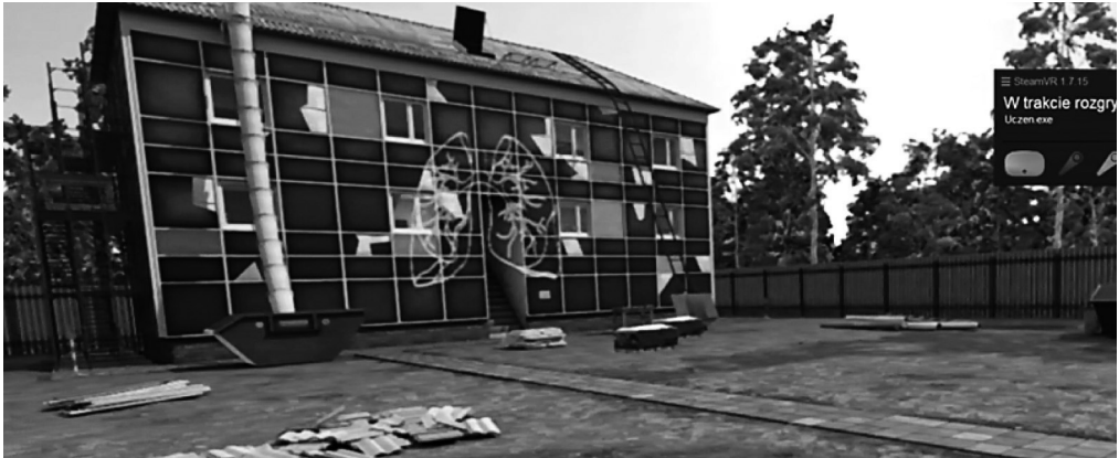
Fot. 3. Screenshot from the VR application – main building where asbestos removal works are carried out
